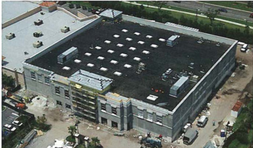
SIKON is building a new Publix Greenwise store at Legacy Place. (Photo by Aerial Photography Inc./www.ap4.com)
